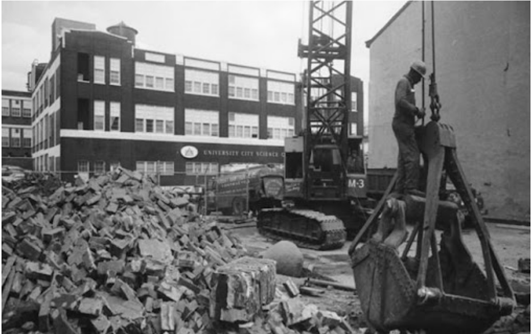
Figure 5. The Demolition of a Building Near the Southwest Corner of 34th and Market Streets, 1967
